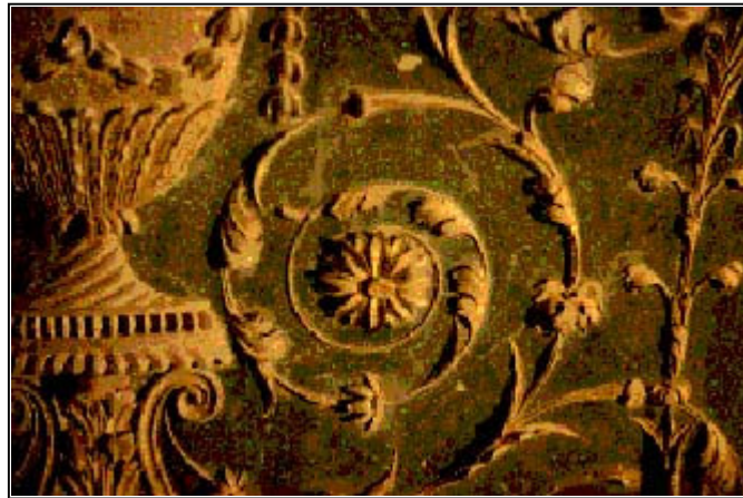
18th century hand modelling at Prior Park executed in marble dust, lime and gypsum.
