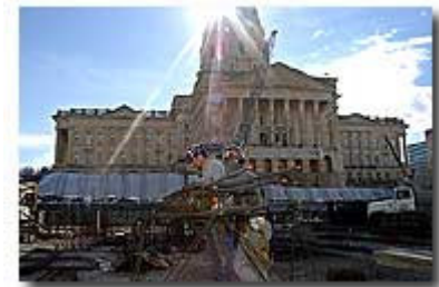
Ed Peel and Matt Myers, of Kaw Valley Steel, work on the rebar for a column of the underground parking garage and visitors center on the north grounds of the Statehouse.
